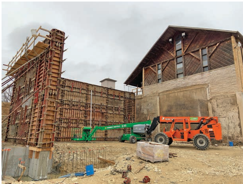
Foundations are being poured for a 4,500-square-foot building addition that will include a warehouse for the new food pantry.
